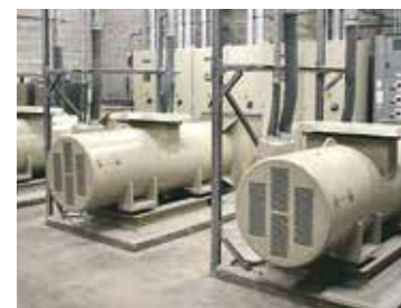
Central system with times-top Motor-Generator Sets.
